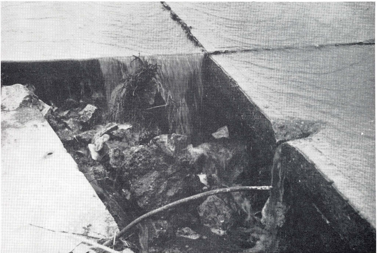
Heavy rains resulted in this damage to the spillway apron in the year 1940. Such occurrences pose a problem of constant maintenance at the State Lakes in Kansas.
